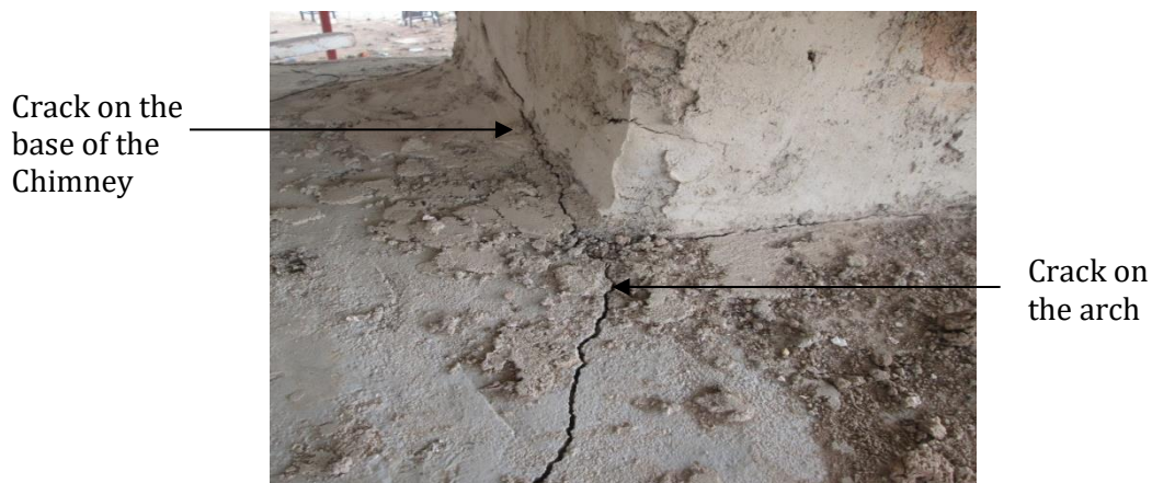
Figure 9. Cracks on kiln arch and chimney base
